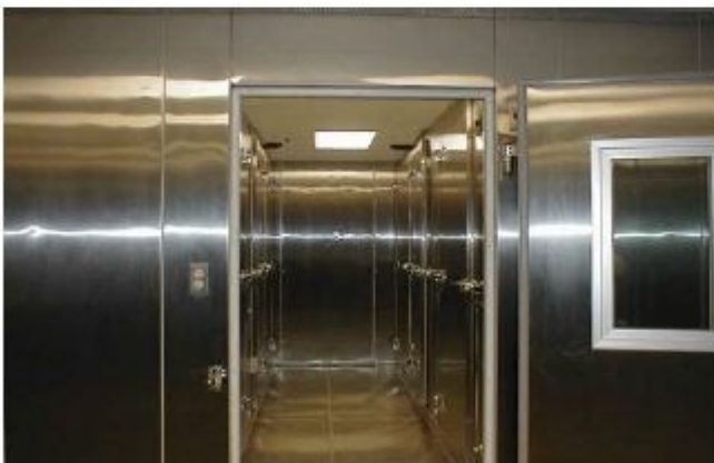
Pictured above – Typical hall with access to multiple cold storage compartments on both sides
